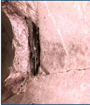
Pipe with hole
