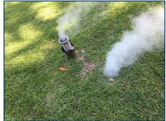
Lateral Defect (Basin 5A) MH0199:MH0197
