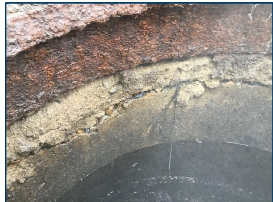
Defective Chimney (Basin 3) MH0336
