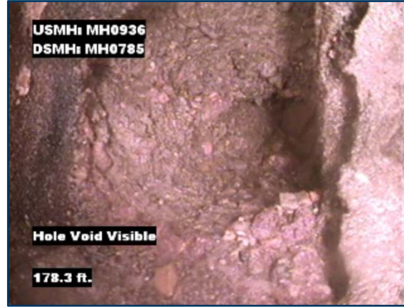
Pipe with hole
